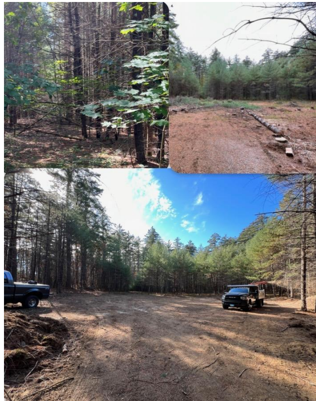
Cemetery & Parks ongoing cremation park project Before (top left), During (top right), Current (bottom)
